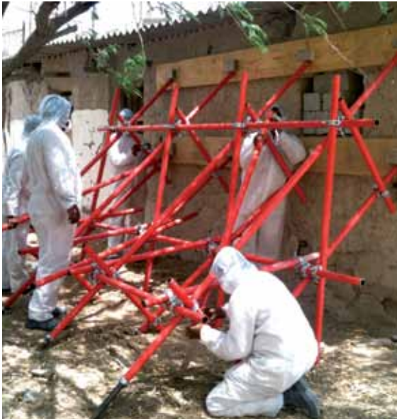
Installing scaffold to support exterior mudbrick wall at Ahmad Bin Hilal al Dhaheri house. The team followed standard environmental safety protocol by wearing protective gear.
