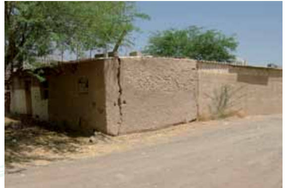
Ahmad Bin Hilal al Dhaheri house with its older traditional mudbrick masonry (left) and its modern concrete block addition (right).
